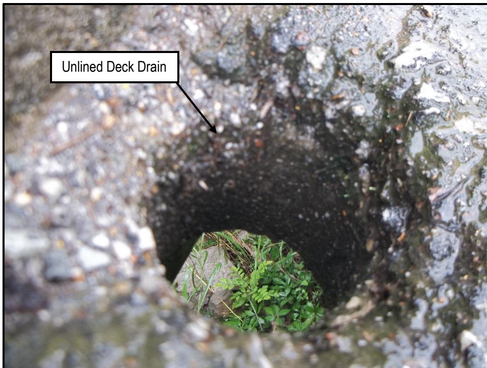
Photo 8: Unlined Deck Drain on SR-436 Bridge over Reedy Creek
